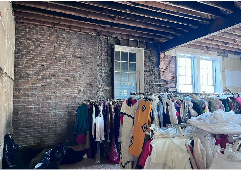
1908 BUILDING - CEILING FIRE DAMAGE
